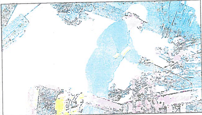
Brad Whiffin, a swamper with TCL, works to secure the trencher in place on a truck.
